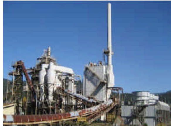
Blue Lake Power Plant: fuel conveyors in front, boiler on left, emissions control in middle, cooling system to right
